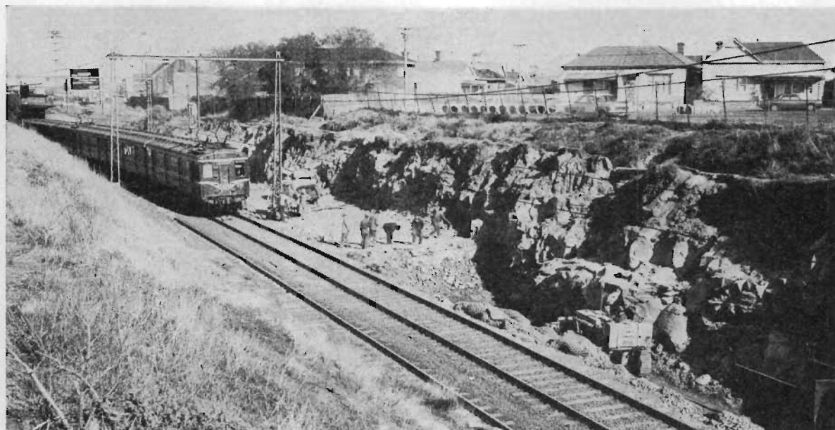
The $5 million project to improve train services to Melbourne's western suburbs and beyond is under way. Two more rail tracks will be provided between South Kensington and Footscray.
