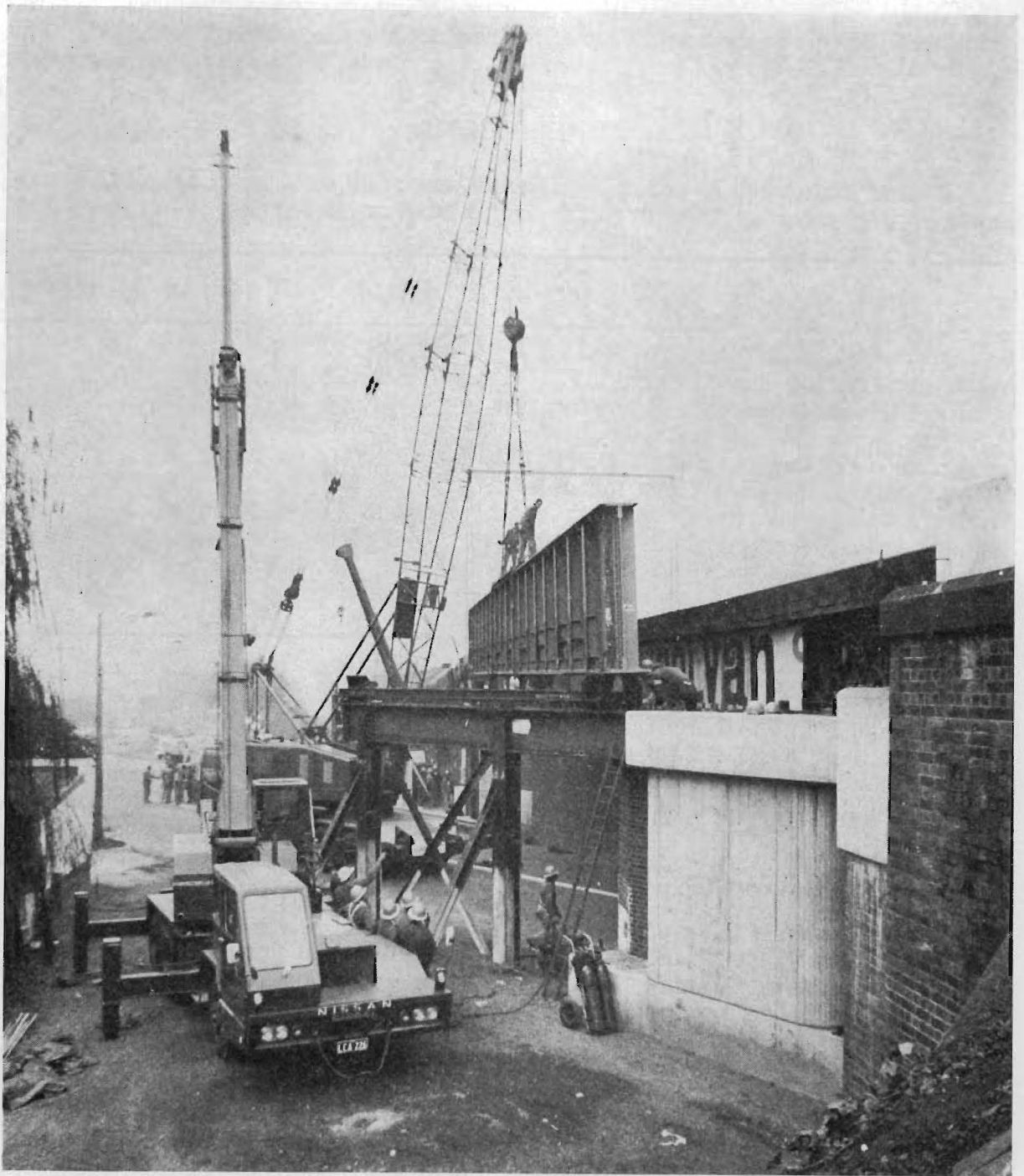
An 150-ton plate girder bridge, 101 ft. long, is being placed in position as part of the reconstruction of the railway bridge over the Nepean Highway at Gardenvale.
