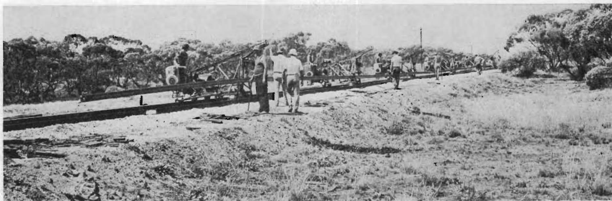
A mechanized gang works on the $6.2 million relaying of the Mildura line.
